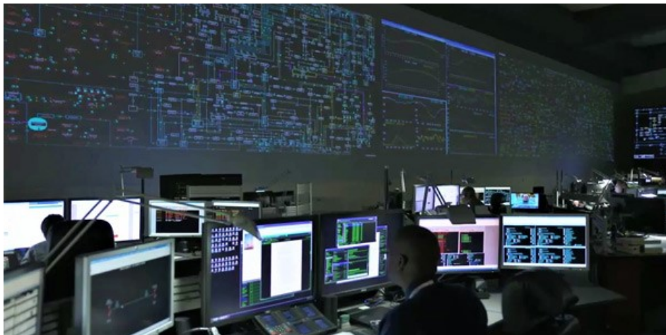
ITC control room | ITC
